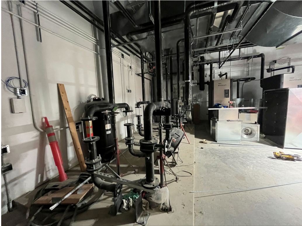
Above: Mechanical Room
