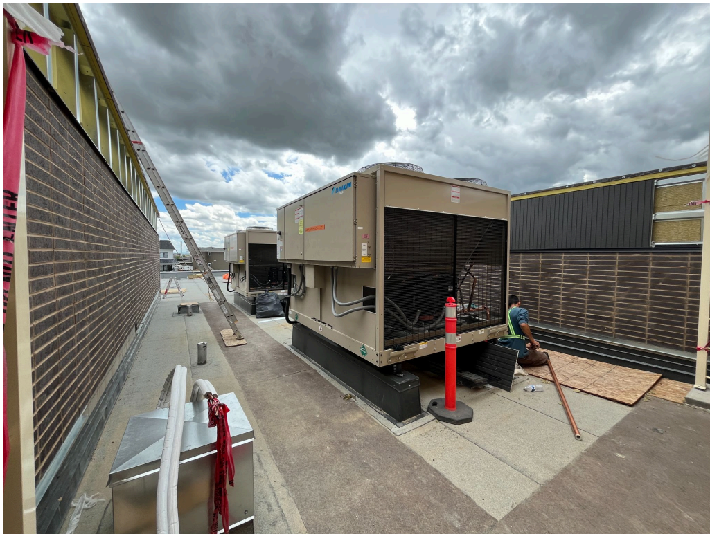
Below: HVAC Equipment on Roof
